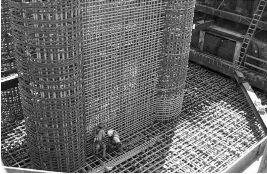
FIGURE 15.13 Overview of footing and pier prior to footing placement. (From Gajda, J., Concrete Technol. Today , 24(3), 34–37, 2003.)
